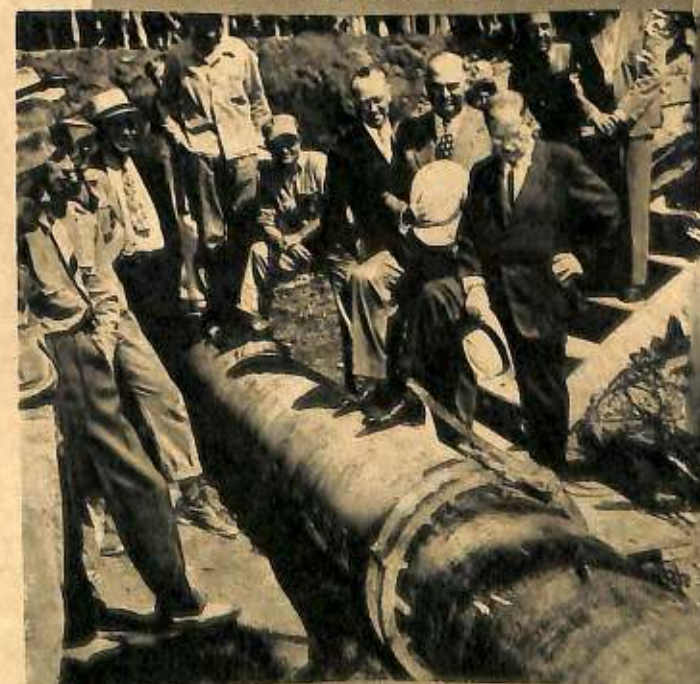
Oil Administrator Harold Ickes looks over the final joint in the Big Inch oil pipe line at Phoenixville, Pa. The pipe will carry 300,000 barrels of oil daily from Texas.
