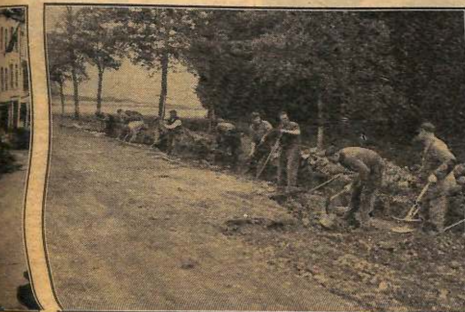
... of the Bulge reached its dramatic climax, the beginning to heal. Belgian civilians clear the debris, a road outside of the town is being repaired.
